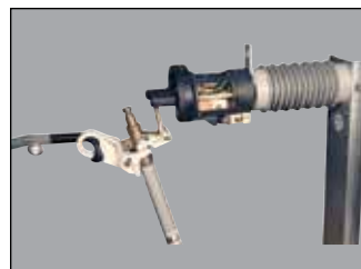
Interrupter parted (internal).
