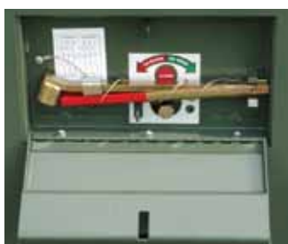
Switch-Operating Handle Storage
