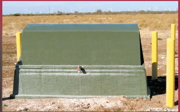
Installed ND-683054 cabinet
